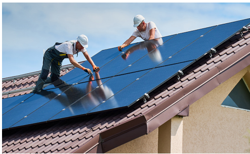
Solar panels turn sunlight into electricity.
